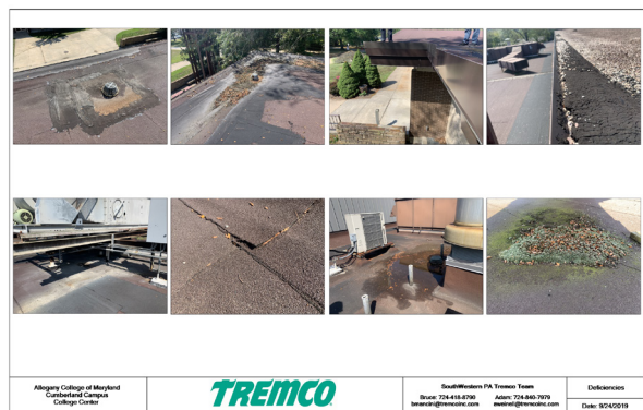
College Center Deficiencies
