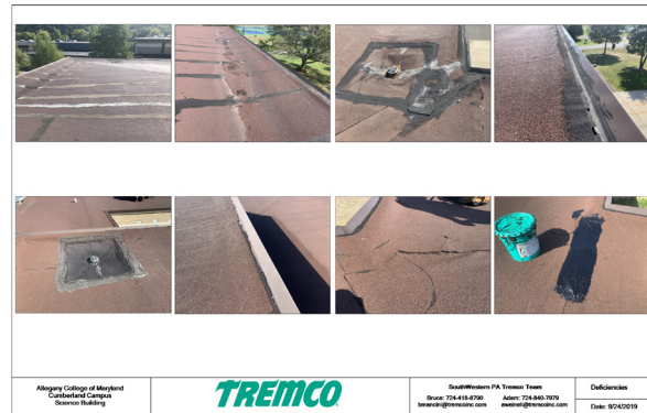
Library Science Building Deficiencies Photos
